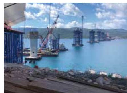
September 2020: View onto the Pelješac peninsula. The bridge is scheduled for inauguration in 2022.
