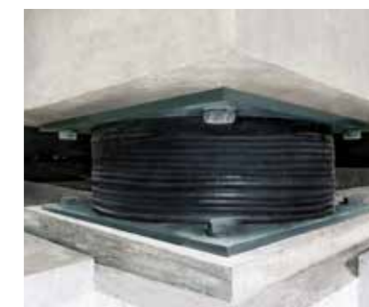
One of the 243 lead rubber bearings between the upper concrete platform and the lower concrete trough. Clearly visible are the ring-shaped deformations of the elastomer due to elastomer-steel plate layering.
